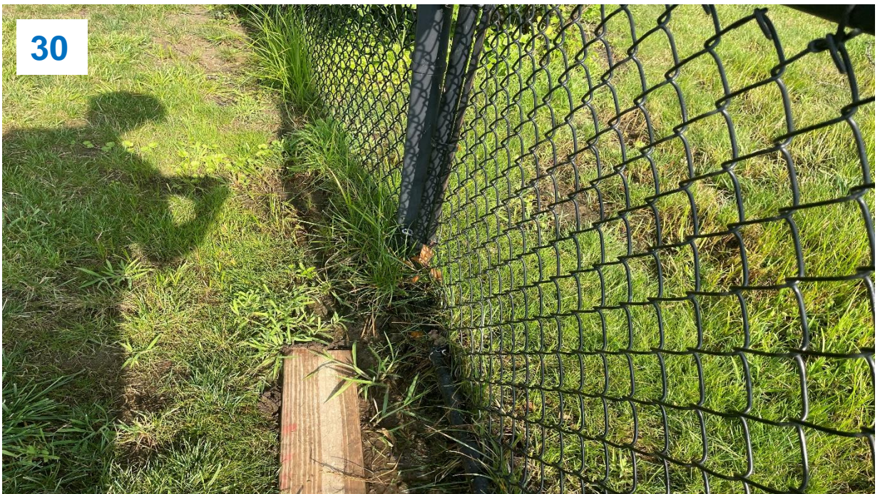
Top: Downstream slope left side, property line fence traversing embankment.
