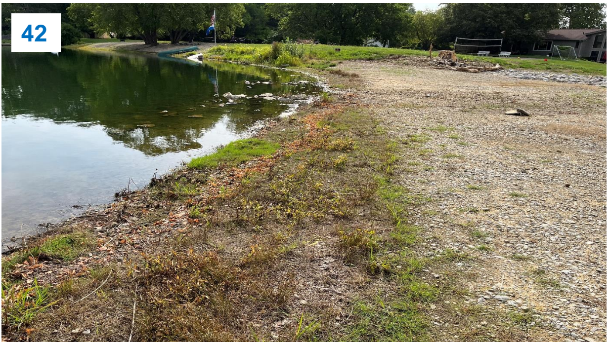
Top: Auxiliary spillway right side, exposed geotextile fabric.
