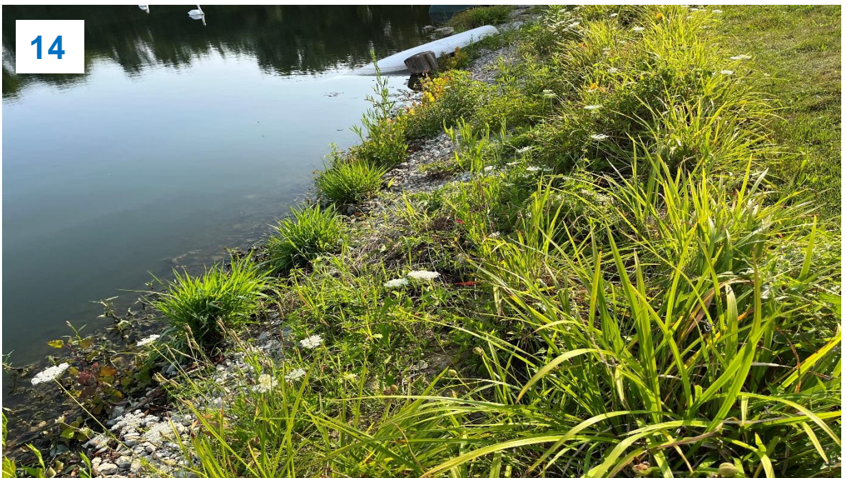
Top: Upstream slope near middle, watercraft, flagpole, and landscaping found on slope.
