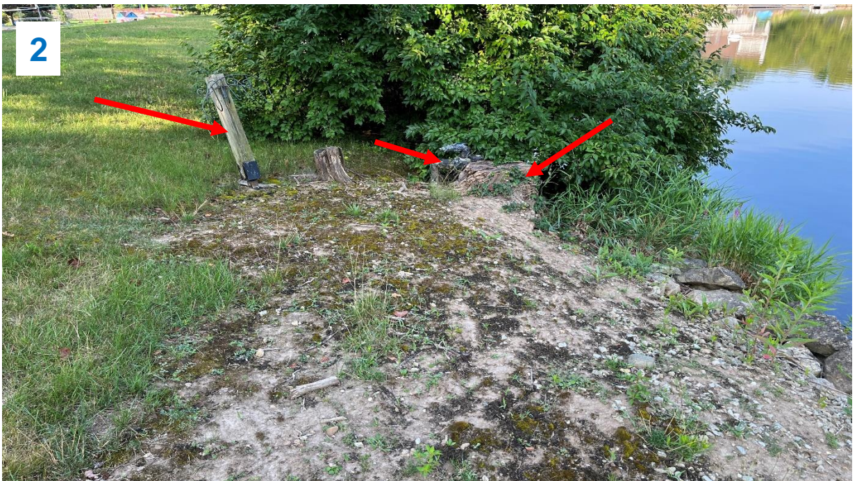
Top: Upstream slope left side. Dock encroaching on upstream slope. Note bare areas and depressions behind dock.
