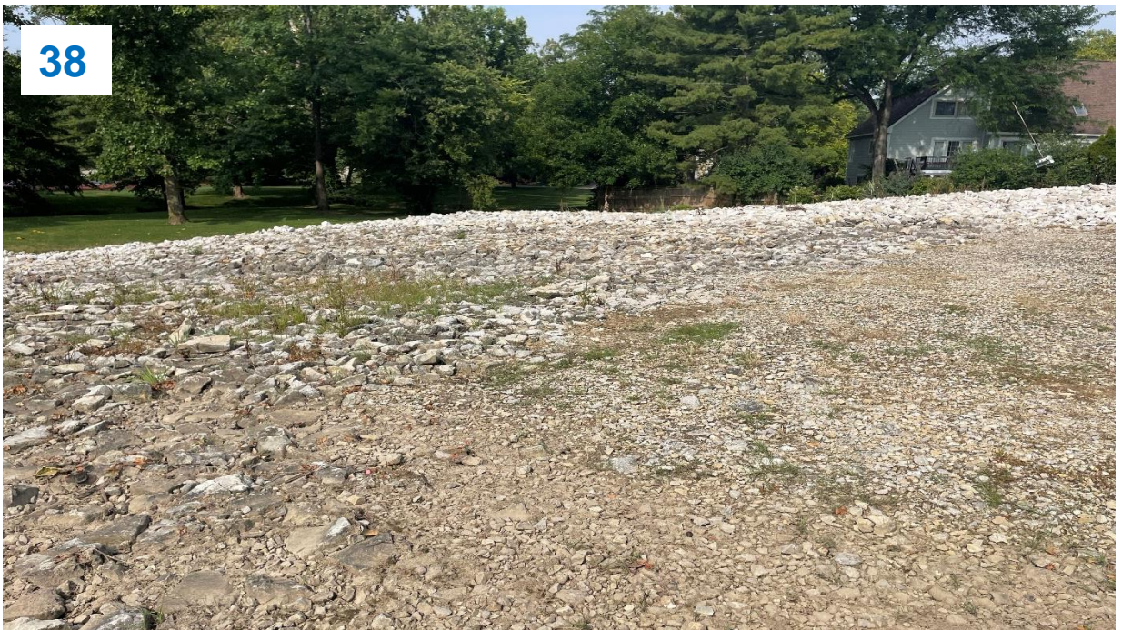
Top: Principal spillway outlet, vegetation in outlet channel.
