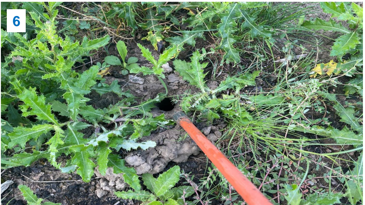
Top: Upstream slope left side. Bare area along fence line.
