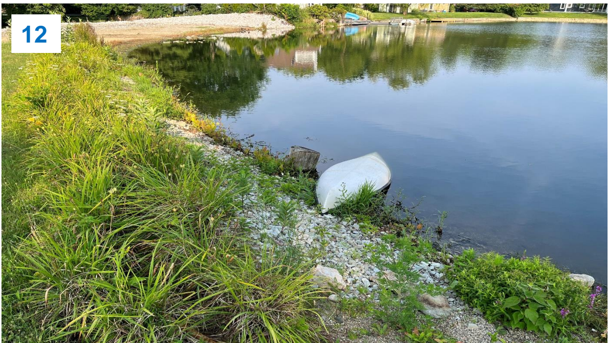
Top: Upstream slope on left side, gravel landscaping, undulating slope, and aquatic vegetation.
