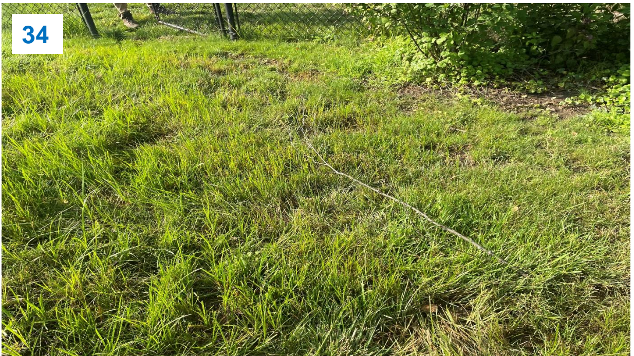
Top: Downstream slope right side, deck with furniture encroaching on slope.
