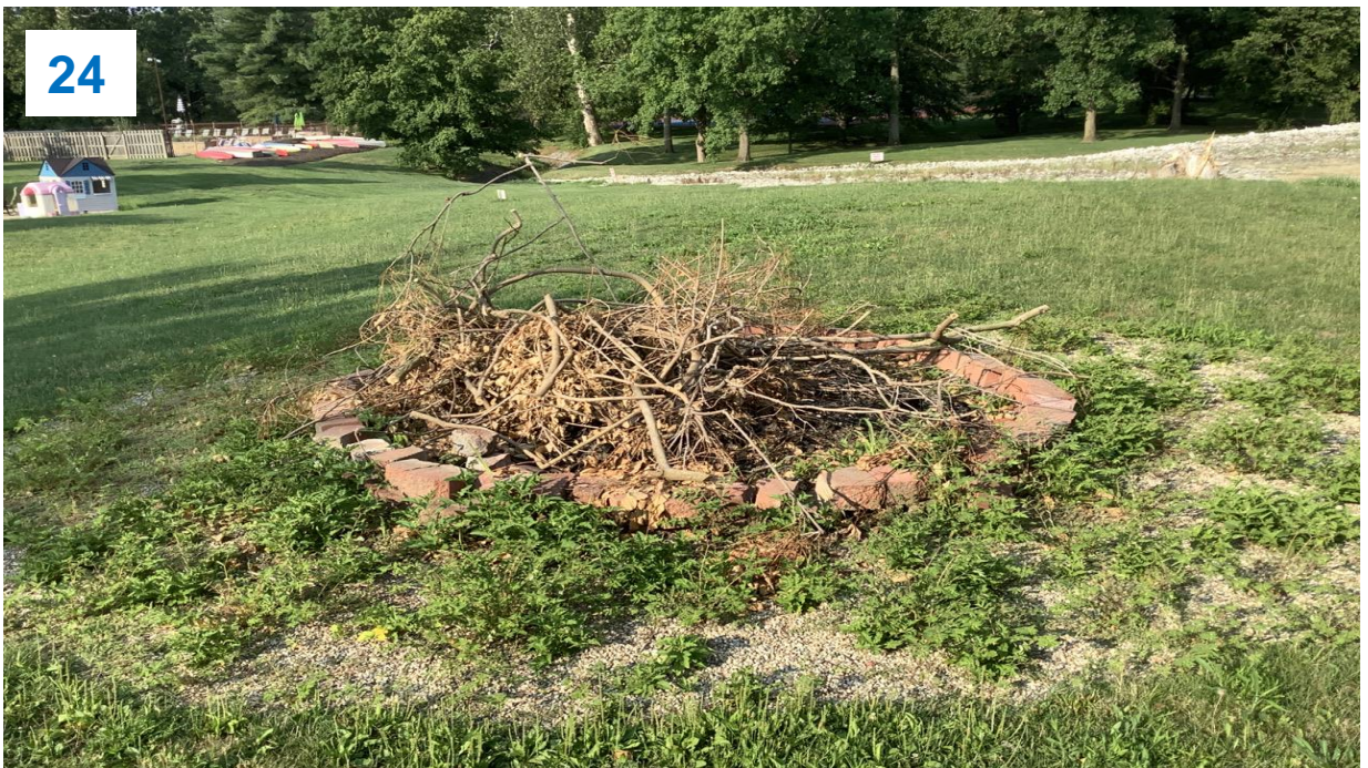
Top: Crest on left side, soft area with tree roots.
