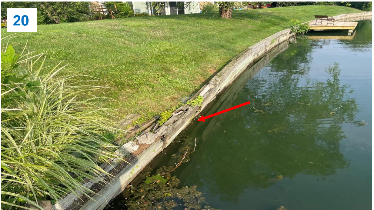
Top: Upstream slope right side, concrete slab cracking and settling into dam.
