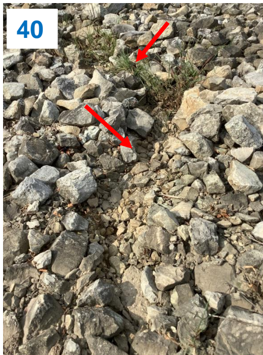
Top: Auxiliary spillway left side, bare area around tree stump.
